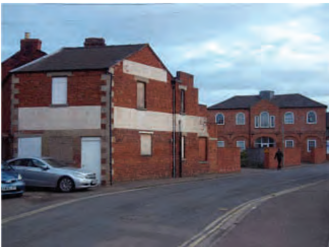
Town Hall wharf, Banbury - in need of some maintenance
