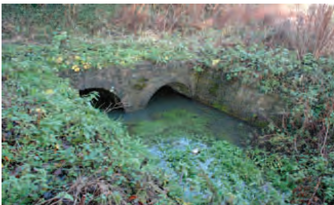
Double arched culvert under the canal at the southern end of a shallow embankment near Clattercote
