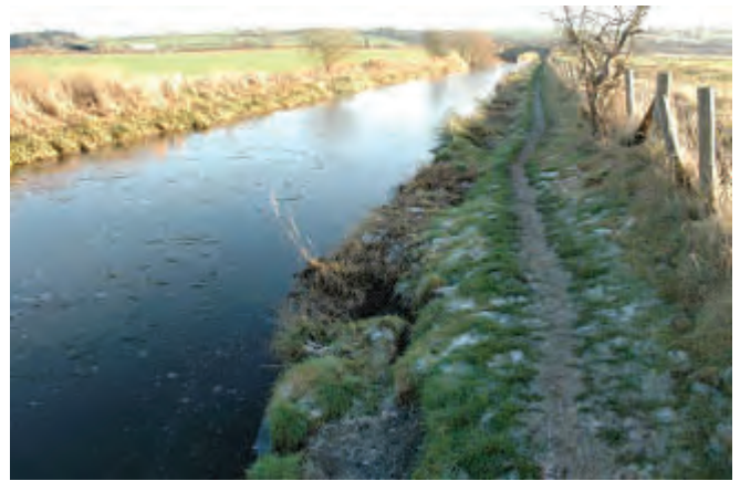
View south from Somerton Deep showing the decayed state of the towpath
