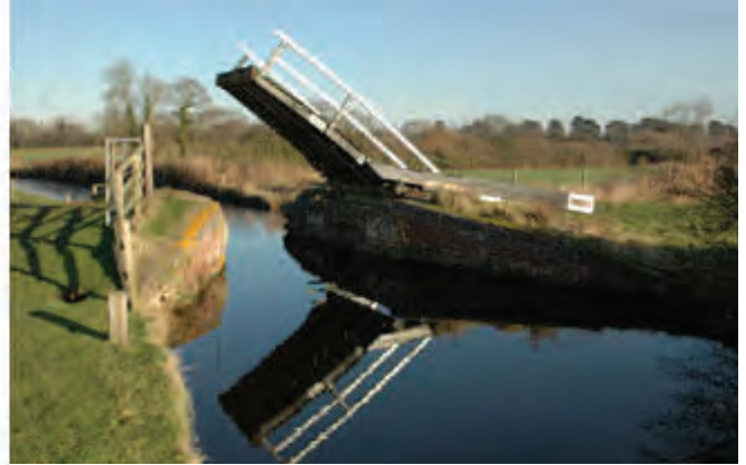
Lift bridge 193 in the raised position ½ mile (800m) from Somerton Deep Lock
